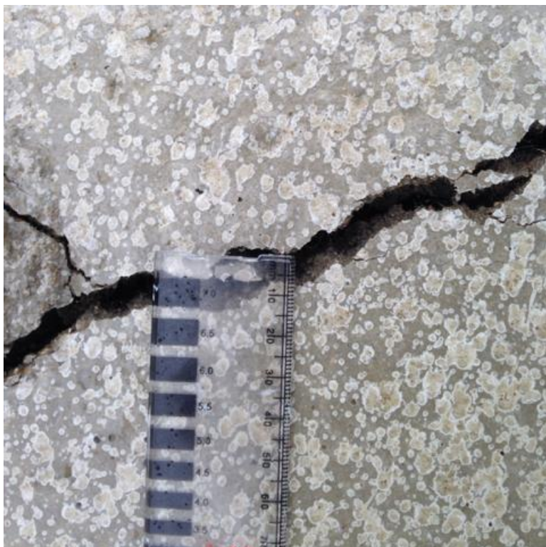
Figure 17 - large crack through the full depth of the hardened slab
